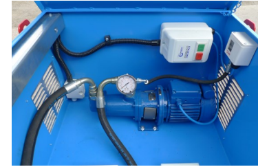
Pump and motor
